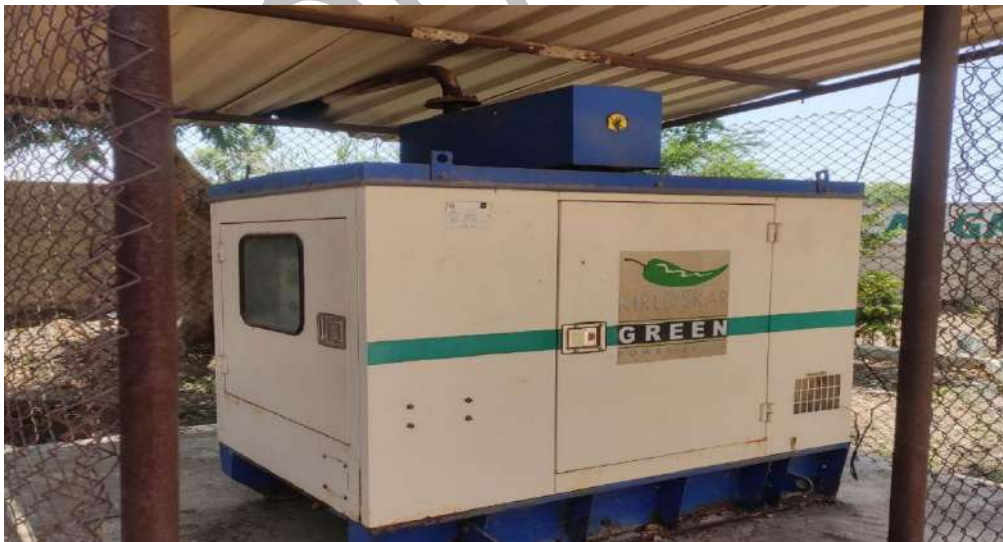
Kirloskar Diesel Generator (15KVA)
