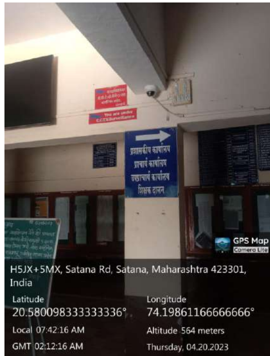
CCTV Camera in Porch
