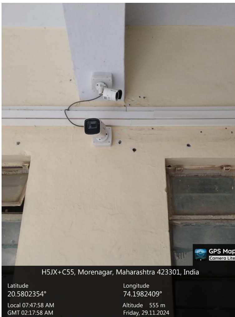
CCTV Camera for Safety and Security
