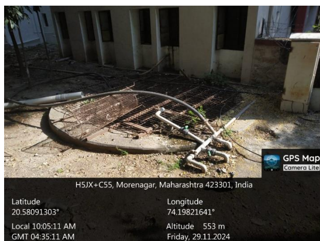
Ditch System for Liquid Waste
